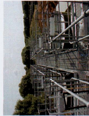
Middlewich WwTW Degremont
